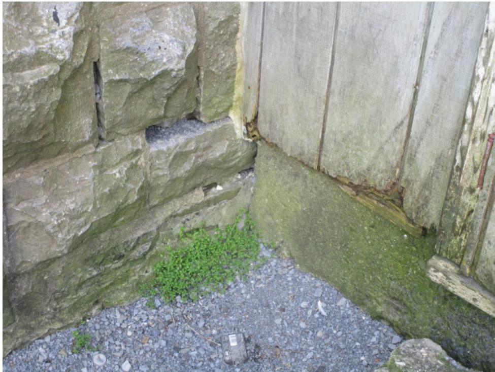
Photo 26 – North-West Addition Siding Deterioration
