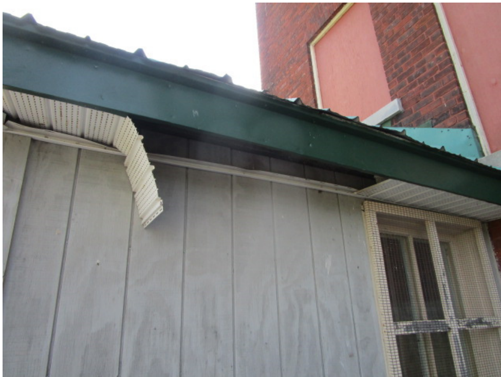
Photo 32 – Damaged Fascia And Soffit
