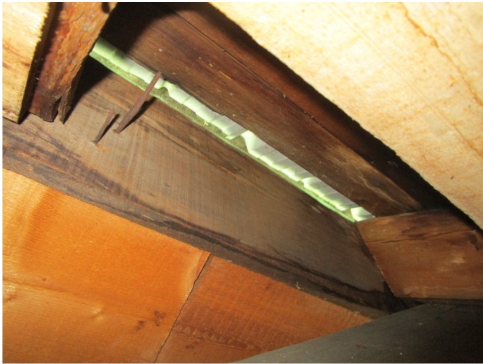
Photo 6 – Suspected Opening In Roof Flashing
