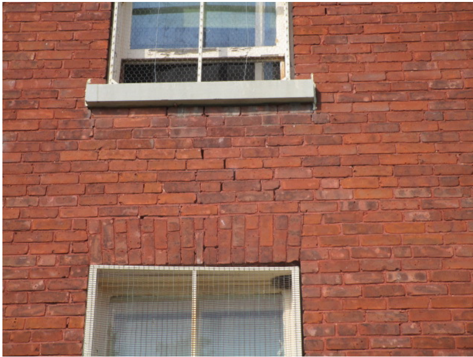
Photo 13 – Brick Masonry Deterioration
