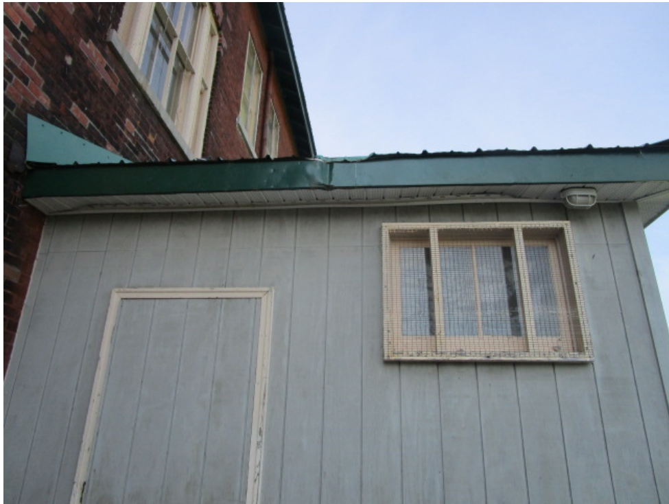
Photo 31 – Damaged Fascia And Soffit
