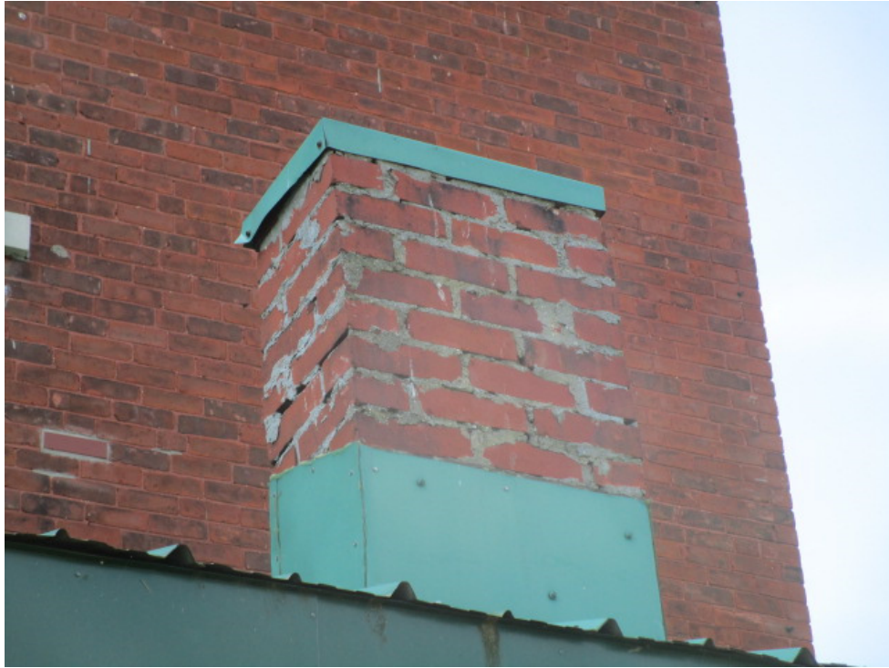
Photo 17 – Chimney Brick Masonry Deterioration
