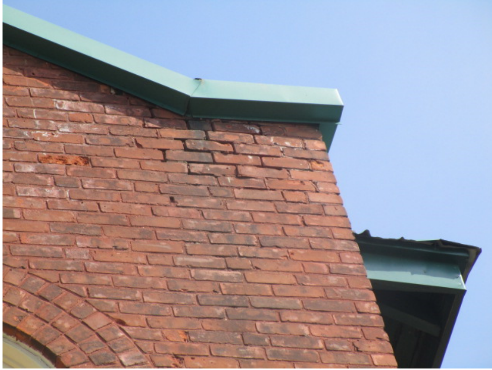
Photo 9 – Brick Masonry Deterioration
