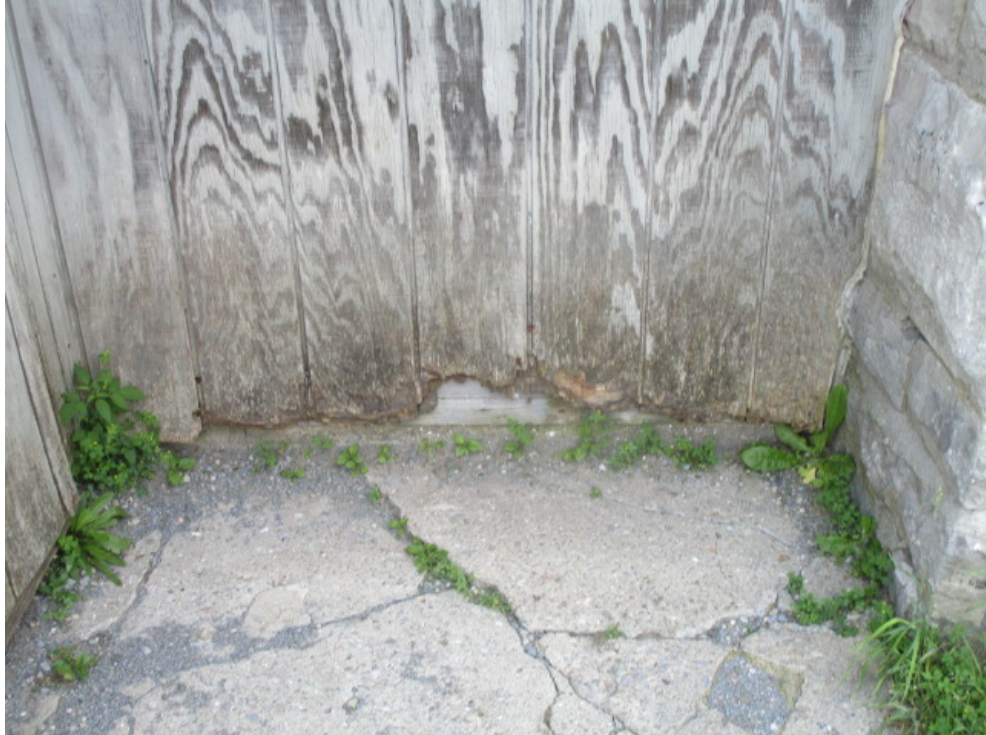
Photo 25 – North-West Addition Siding Deterioration
