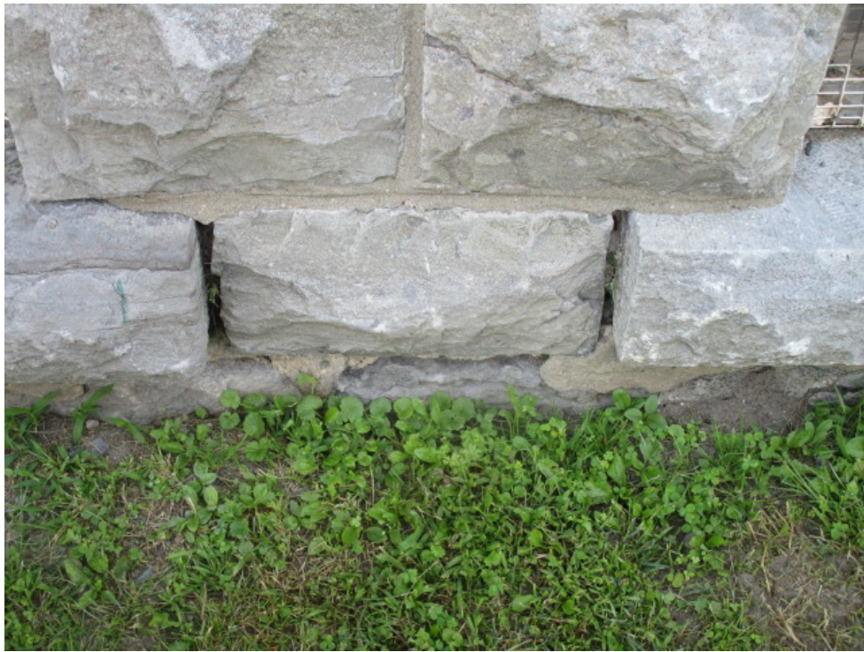
Photo 14 – Stone Masonry Deterioration
