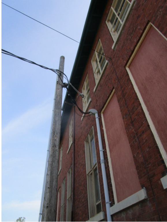
Photo 35 – Dislodged Pole Anchor
