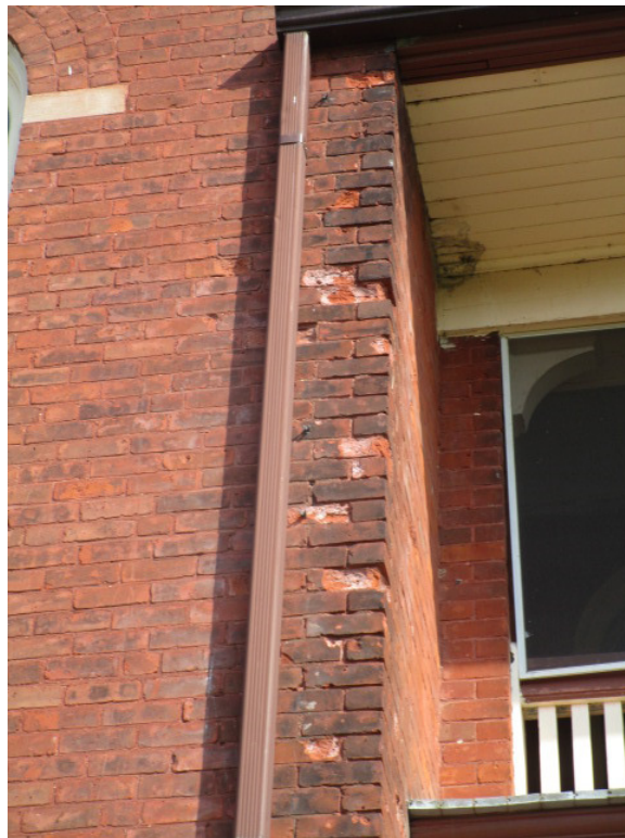
Photo 8 – Brick Masonry Deterioration
