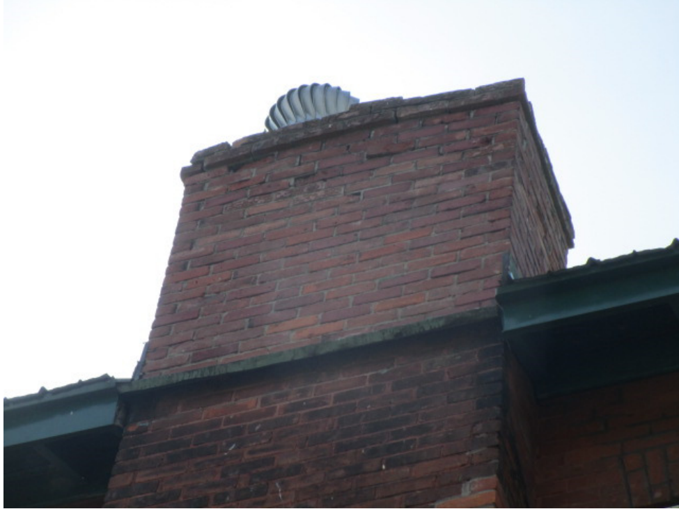
Photo 19 – Chimney Loose Brick Masonry
