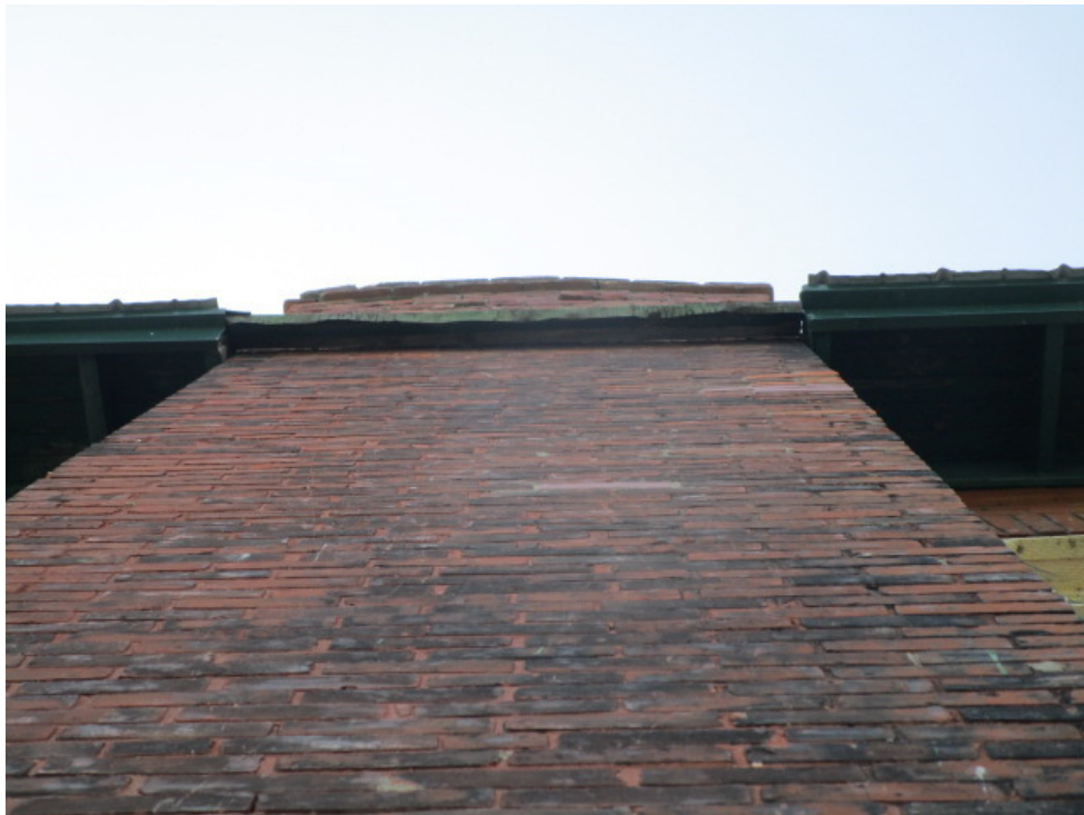
Photo 20 – Chimney Loose Brick Masonry
