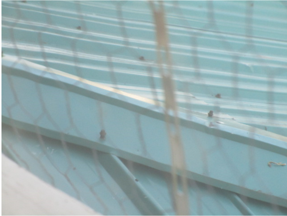
Photo 5 – Loose Roof Panel Fasteners
