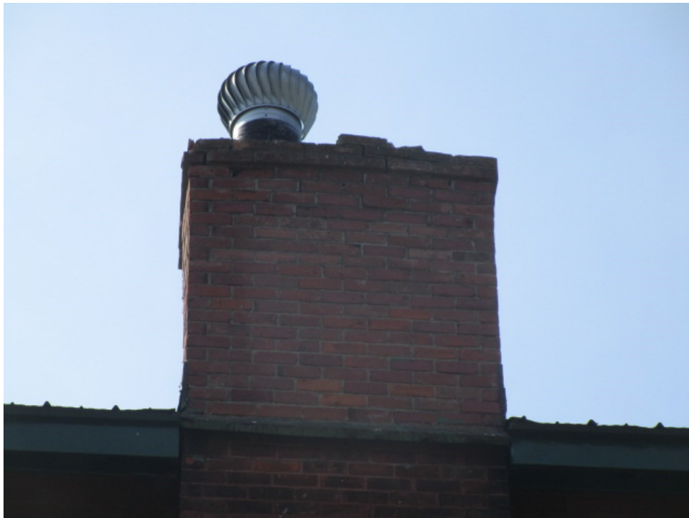
Photo 16 – Chimney Brick Masonry Deterioration
