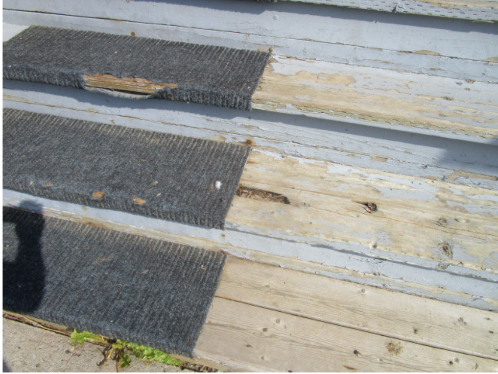
Photo 23 – Front Entrance Stair Condition
