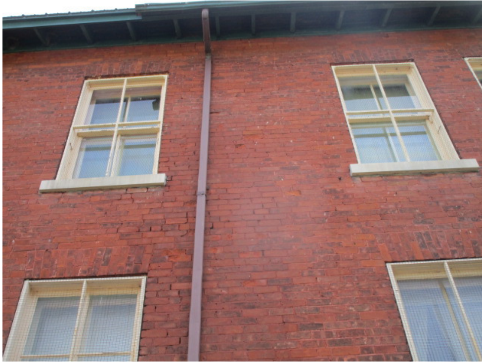
Photo 11 – Brick Masonry Deterioration
