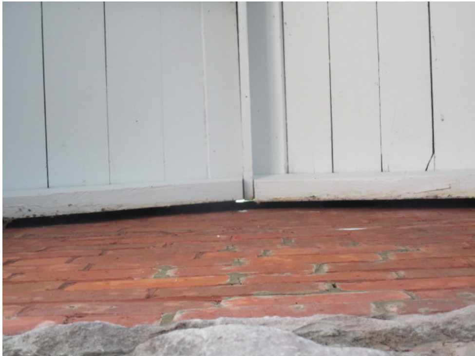
Photo 34 – Suspected Opening In Roof Flashing At North-East Entrance
