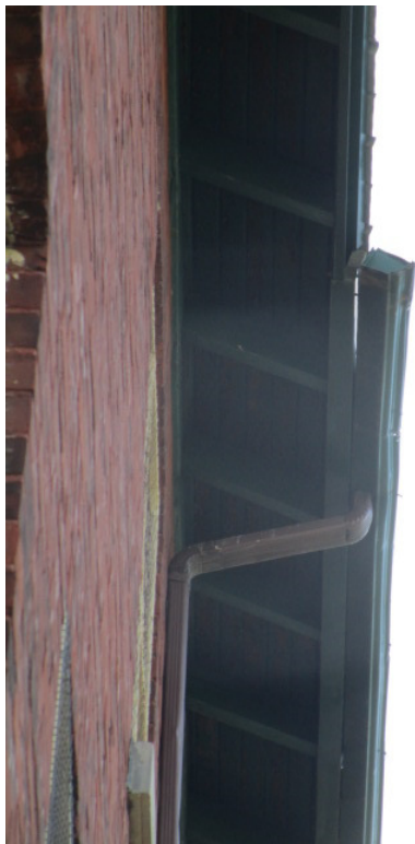
Photo 30 – West Dislodged Eavestrough
