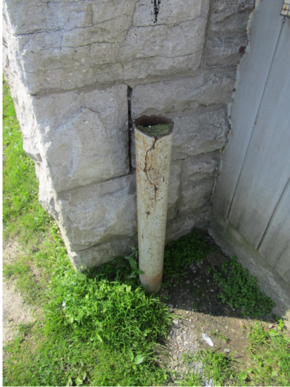
Photo 27 – Former Drain Pipe At North-East Corner
