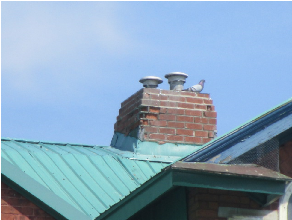
Photo 18 – Chimney Brick Masonry Deterioration
