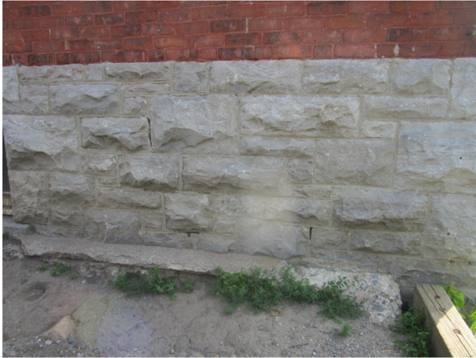
Photo 15 – Stone Masonry Deterioration
