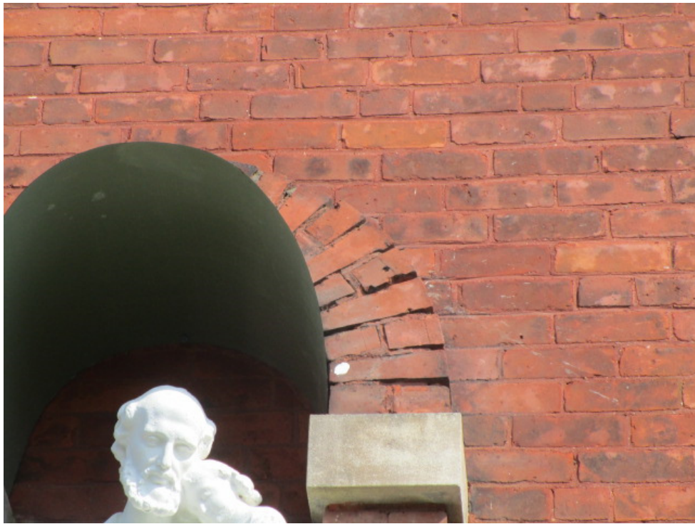
Photo 10 – Brick Masonry Deterioration
