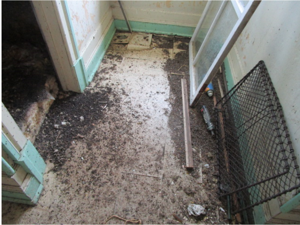
Photo 33 – Third Floor Batt Droppings
