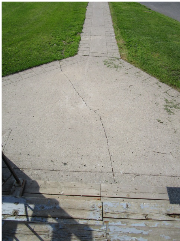
Photo 28 – South Entrance Slab Cracking
