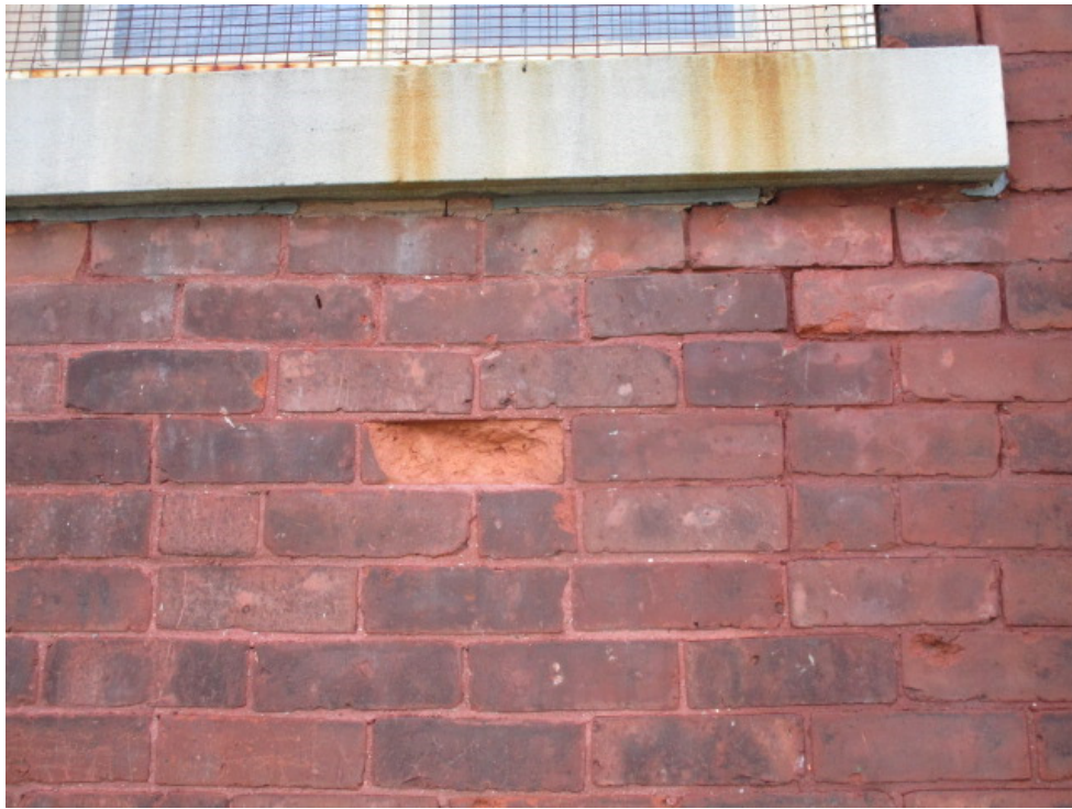
Photo 12 – Brick Masonry Deterioration
