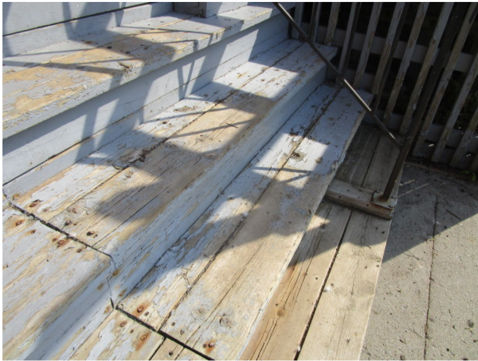
Photo 24 – Front Entrance Stair Condition
